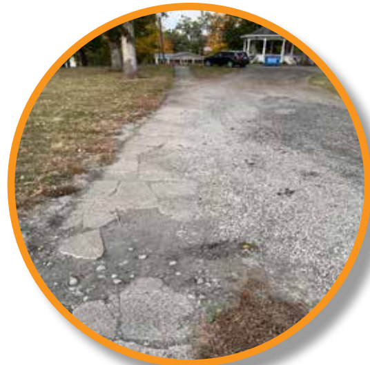
Areas of sidewalk are broken and eroded along primary routes
