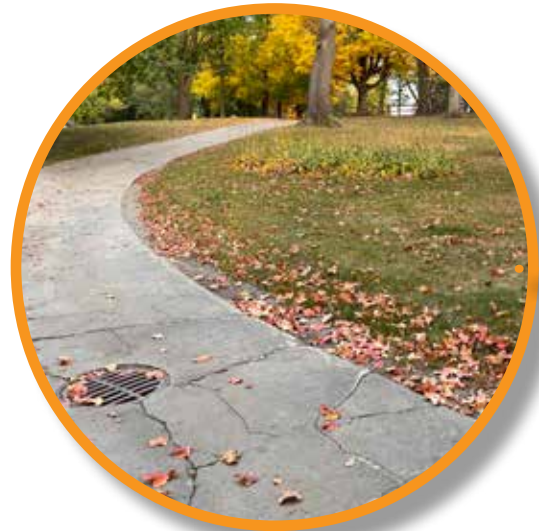
Water flows down the hillside into the driveway, which acts as a swale; erosion is occurring at the edges of the drive
