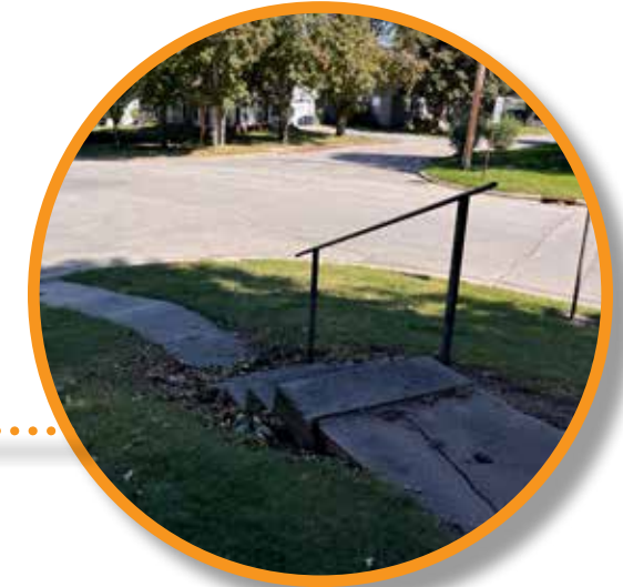
Northeast entry has limited accessibility due to aging stairs
