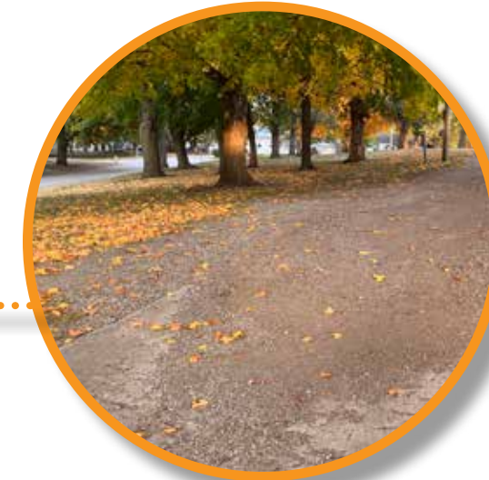
Lack of an edge to the parking lot is allowing the gravel to wash down the hill to the north
